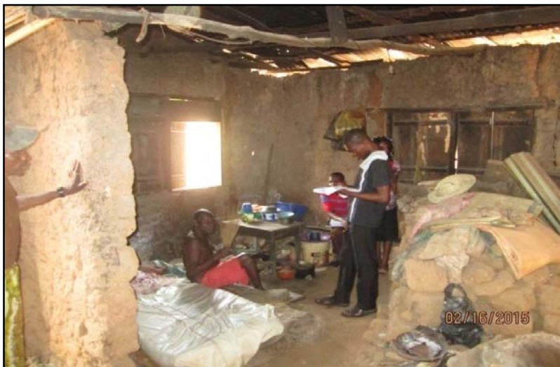
Plate 1: An inhabited dilapidated house caused by flyrock and vibration at Lamulo village, located few meters from a quarry site in Oluyole LGA. Oyo State
