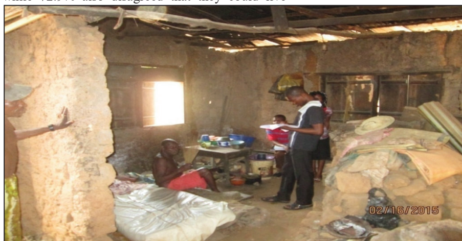
Plate 1: An inhabited house whose dilapidation was caused by flyrock and vibration at Lamulo village, located few meters from a quarry site in Oluyole LGA. Oyo State
